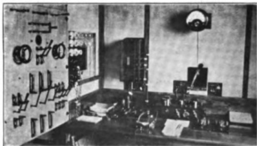
Instrument Room showing Switchboard, etc.
