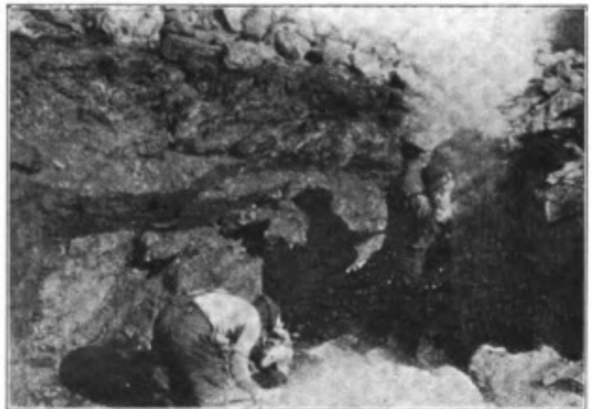
Blasting a hole in the rocks for the foundations of one of the masts.
