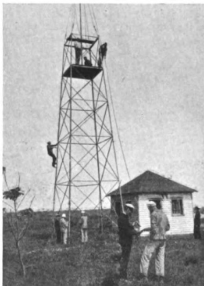
Photo by Sports and General Constructing a Wireless Telegraphy and Telephony Station at Roosevelt Field, Mineola, for the Reception of the R.34.
