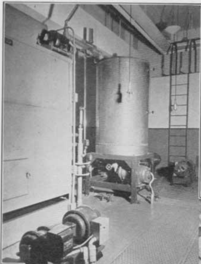
FIG. 36. ABOVE, WATER COOLING EQUIPMENT FOR THE ULTRA-FREQUENCY TRANSMITTING TUBES. THE ROUND TANK IS FOR STORAGE, WHILE THE RECTANGULAR TANK IN THE FOREGROUND CONTAINS THE COOLING UNIT.
