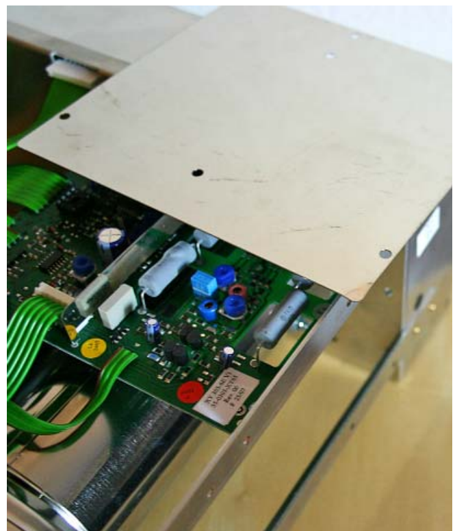
Cabinet capacity replacement
