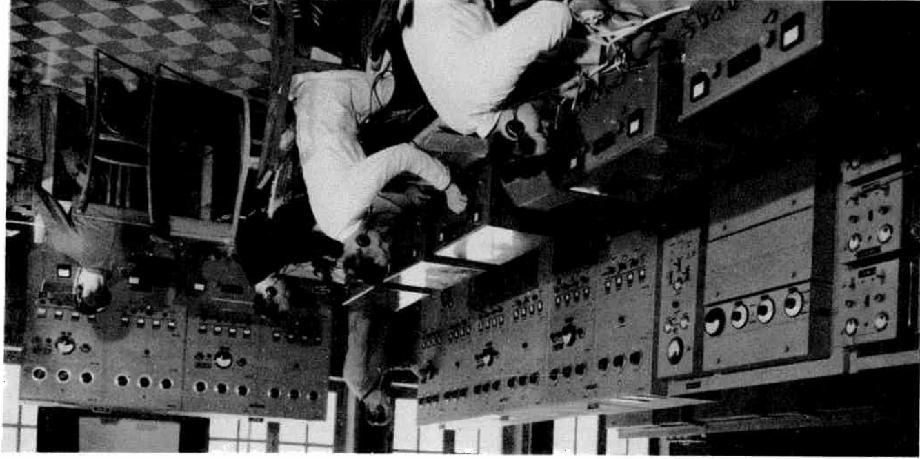
Traffic room fitted with stabilidyne receivers.
