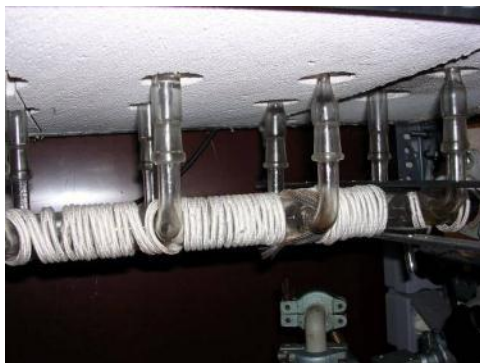
27 Vacuum rack with glass joints
